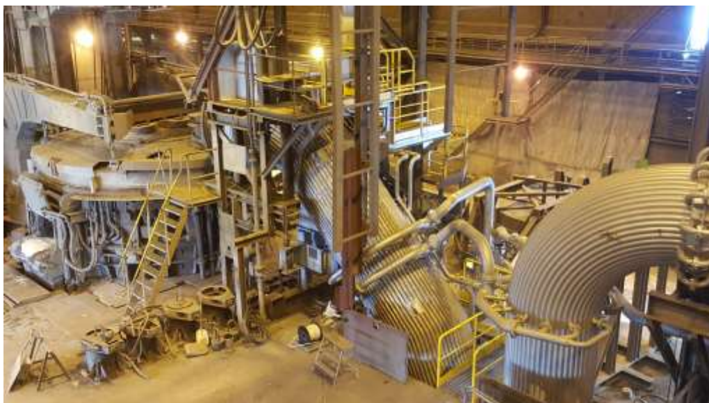
The modernized primary gas cooling system by SMS group at the electric arc furnace of Uddeholm.
