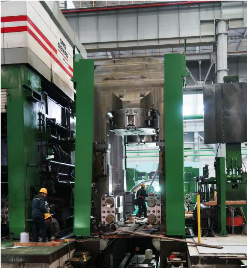
Installation of the new mill stand in position F1 of the finishing train.
