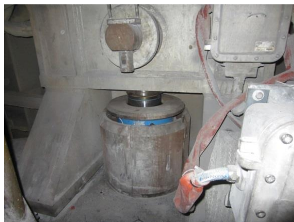
Load cell protection box on the platform
